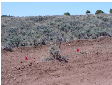
Each lot is marked for placement of the water meter and hookup
