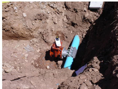
Connection into Main Water Line
